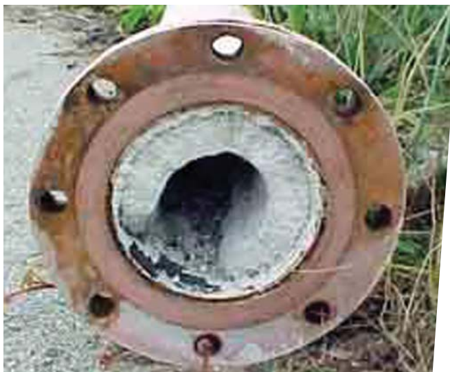
Section of Sewage pipe clogged with phosphorus-rich struvite
