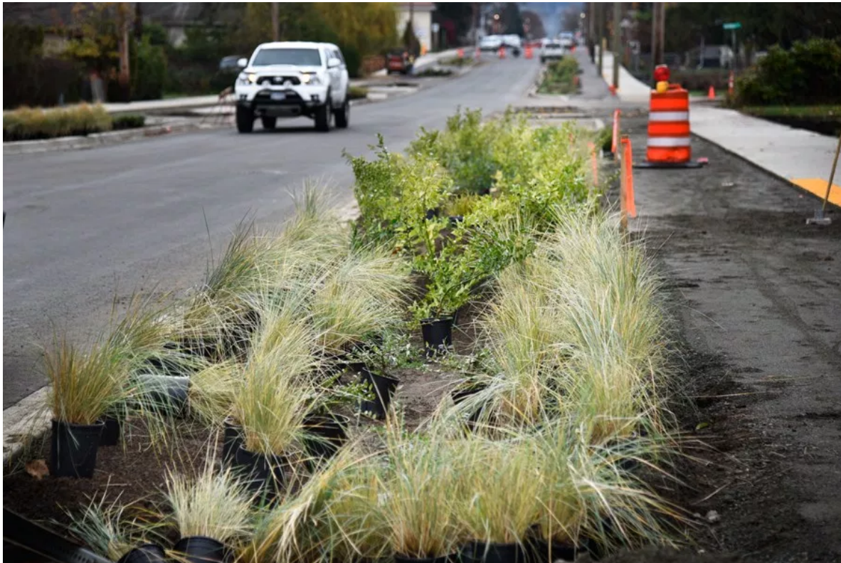
Grasses ready to plant in the rain gardens that line Courtenay's Fifth Street renovation. George Le Masurier photo
