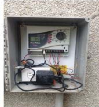
Controller Controller wiring should be cleaned up and a new controller with Monthly Seasonal adjust should be installed.
