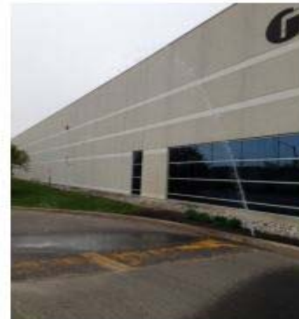
zone 3 damage caused by lawn maintenance
